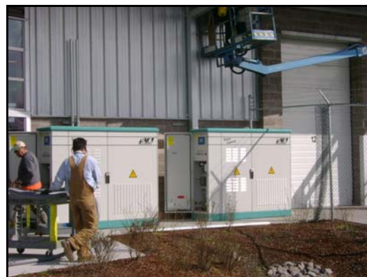
Two of the inverters used to convert DC power output to AC power
